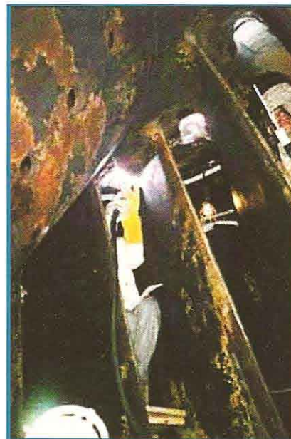
Fig. 1. Welder between the blades of a hydraulic turbine in a power generation unit.
